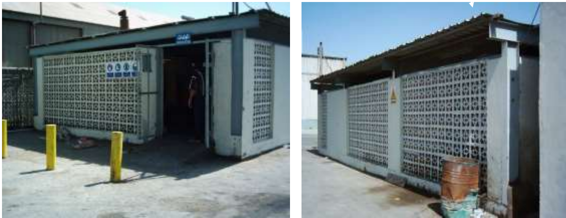
Fig. 1.: Present generator room, Aden Cement Enterprise
